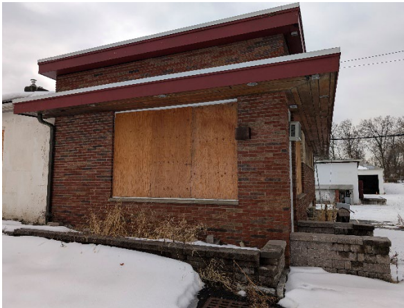
View of the boarded-up office window.
