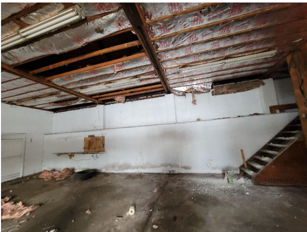
View of a storage room located at the rear of this building. This storage room contains a loft that is used to store planks of plywood or other related materials.
