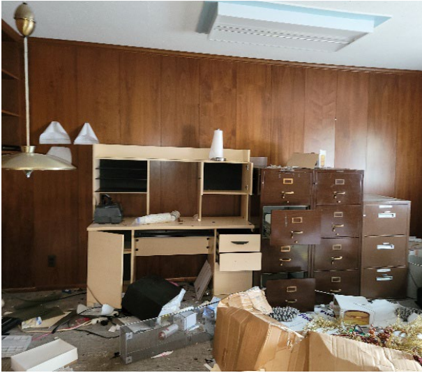
View of one of the offices that has been falling into disrepair and vandalized.
