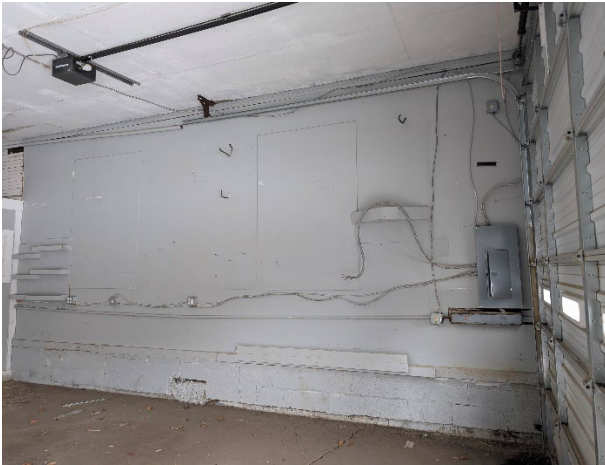
Above Left: Interior view of Building D that shows exposed wiring and an electrical box.
