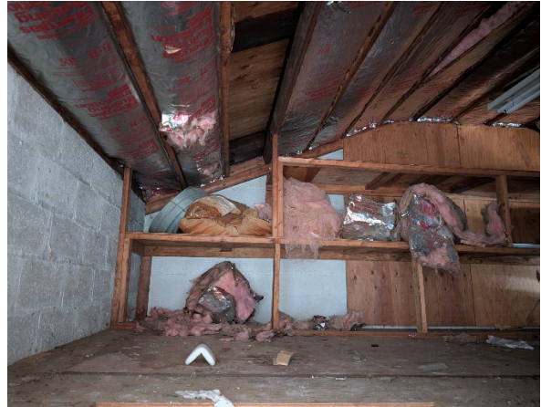
An additional close-up view of the trash and debris.
