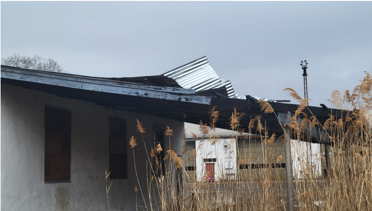
A closeup view of the roof of Building D showing the metal roof.
