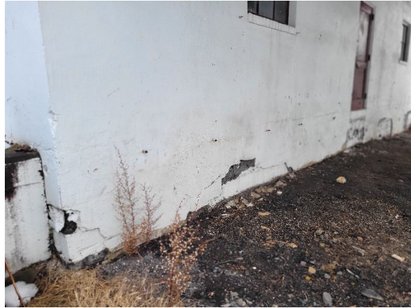
A close-up view showing signs of deterioration.
