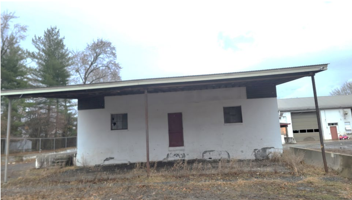
View of the south facing side of Building C. There are no stairs leading to the side doorway and the gravel/asphalt surrounding the building is completely overgrown. The windows are broken on this side but are not boarded up.
