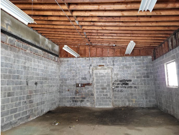
Image of the interior of Building C illustrating signs of mold and water damage on the floor and walls.
