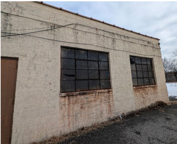
View of dilapidated windows and deteriorated conditions on the side of the building.
