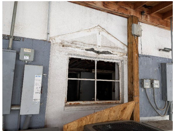
A close-up view of the shattered window near the building's side entrance.
