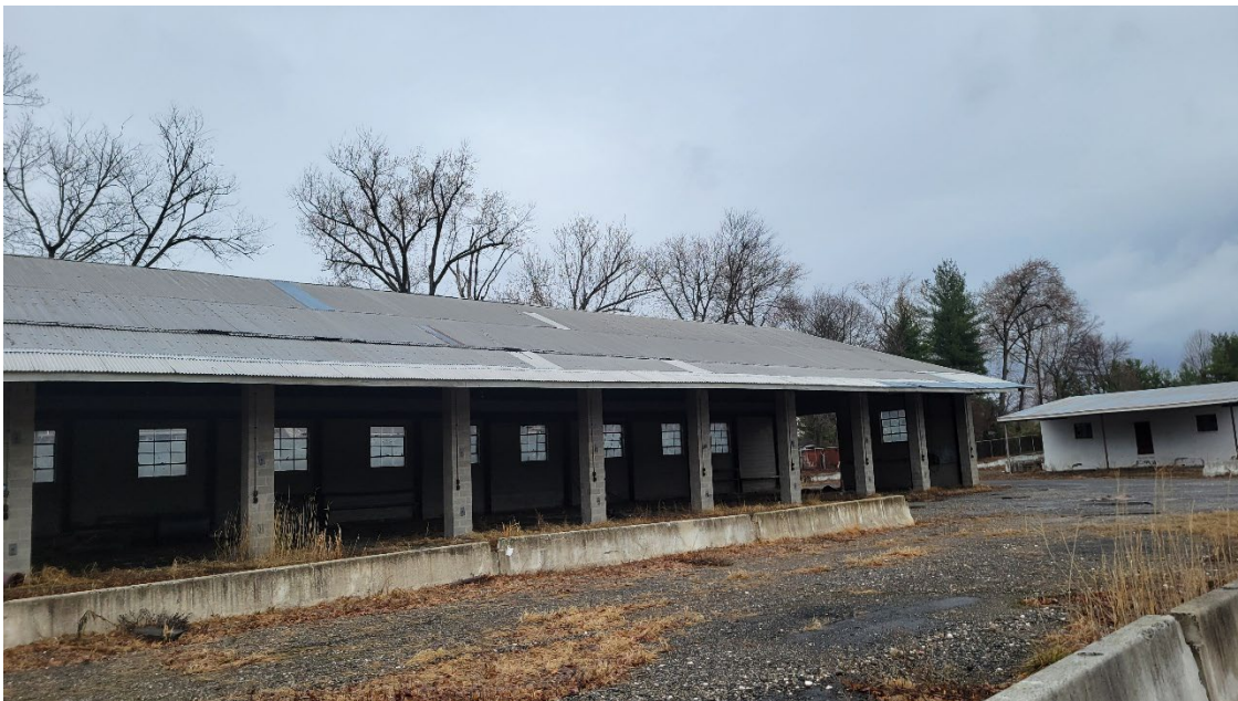
A view of Building E with Building C in the background, to the right. The southeasterly side of building E is open to the elements and is deteriorated. The area between the concrete barrier blocks is fully covered in gravel.
