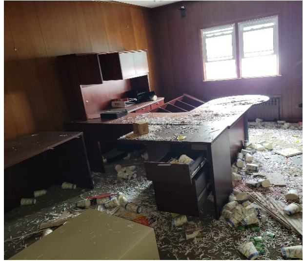
Another office that has trash and debris all over the floor, showing more signs of potential vandalism.
