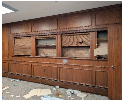
Further signs of vandalism and/or squatters that have left trash, glass, and paper all over the floor.
