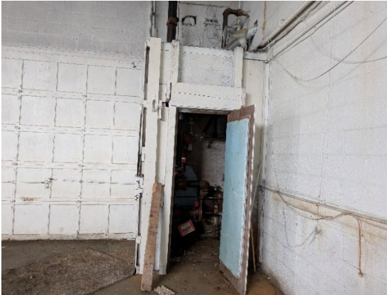
View of the utility closet in Building A.
