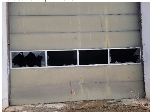
Close-up image of one of the garage doors with smashed windows.
