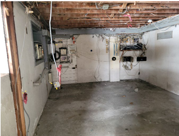
Exposed wiring and utilities that were found in the second building.
