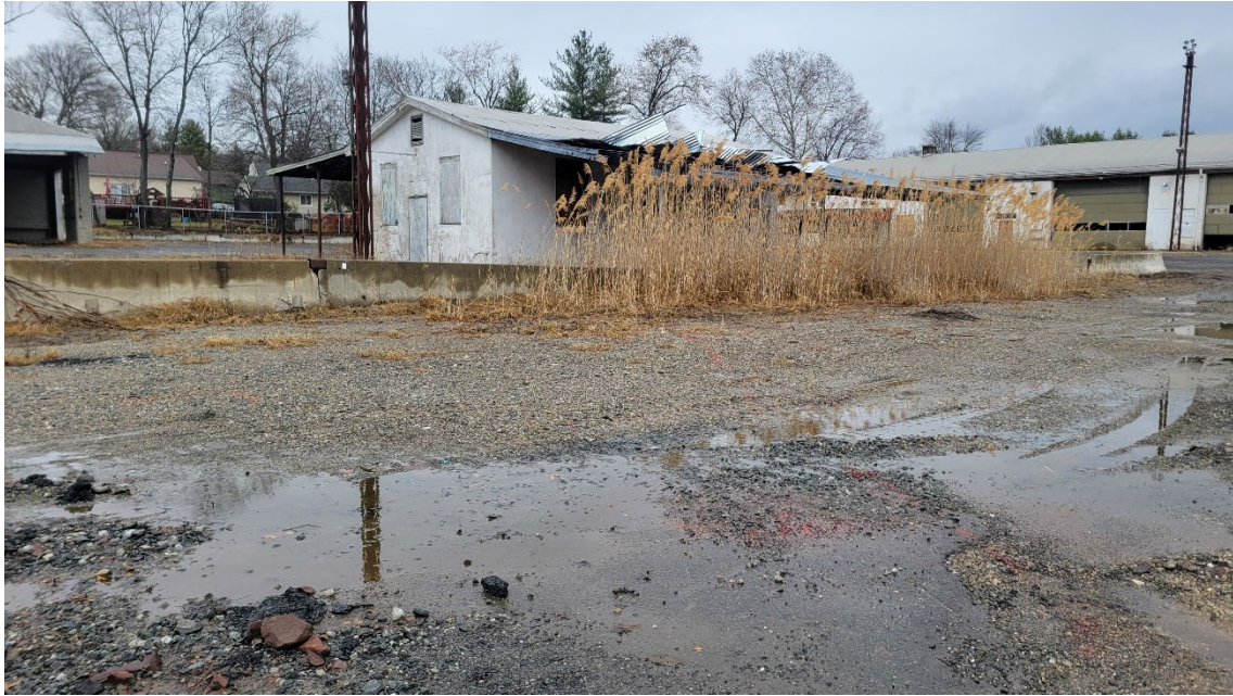
A view of the southeasterly side of Building D where the roof is tearing off. The roof was intact during the site visit on February 19, 2026, less than a month before this visit. This suggests that the property is quickly deteriorating as it is not being maintained.
