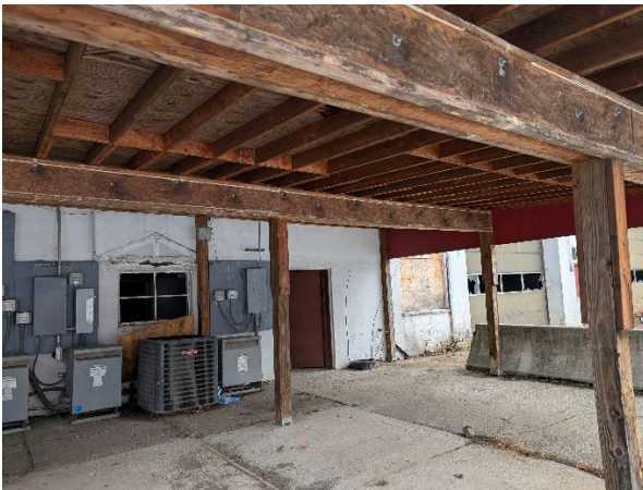
Side entrance depicting a broken window and a boarded-up window.
