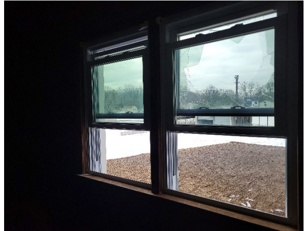
A broken office window that has not been boarded up.
