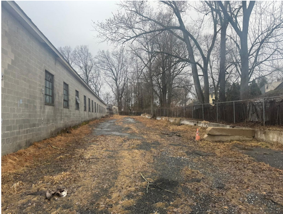
A view of the area to the rear of Building E. The pavement is deteriorated and overgrown. Some of the windows are broken but they are not boarded. Also visible are the single-family homes on the other side of the chain link fence.
