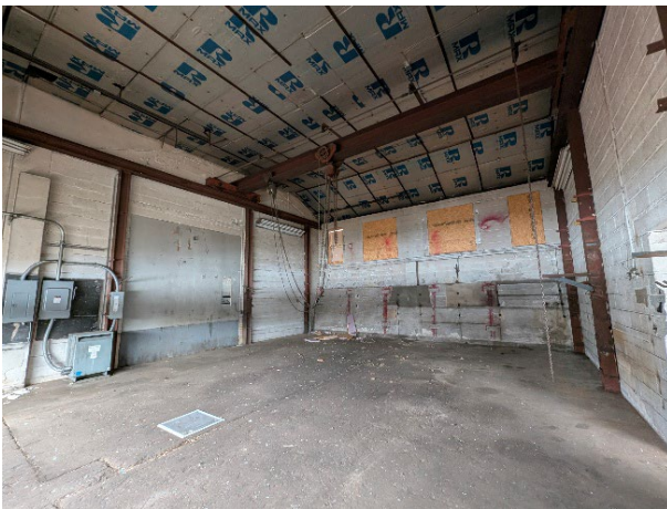
View of the second garage bay with boarded up windows
