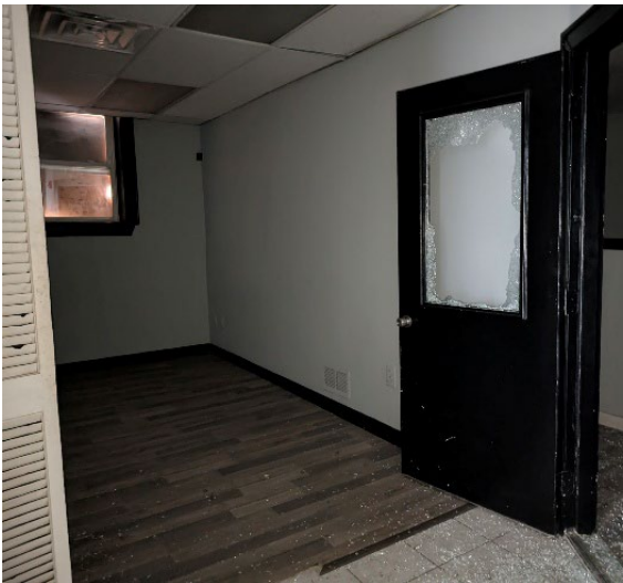
Above Left: Doorway to offices that have been broken into. Further evidence of vandalism.
