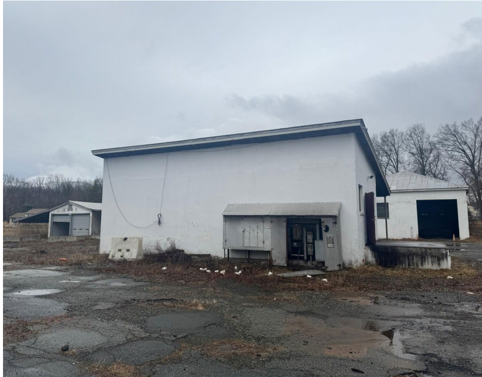
A view of the westfacing side of Building C. Water from recent rain event in the broken and cracked pavement, indicating decline and poor drainage in this area.
