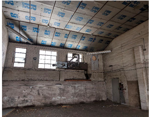
A more detailed view of the interior of the same garage with debris and plywood scraps on the floor.
