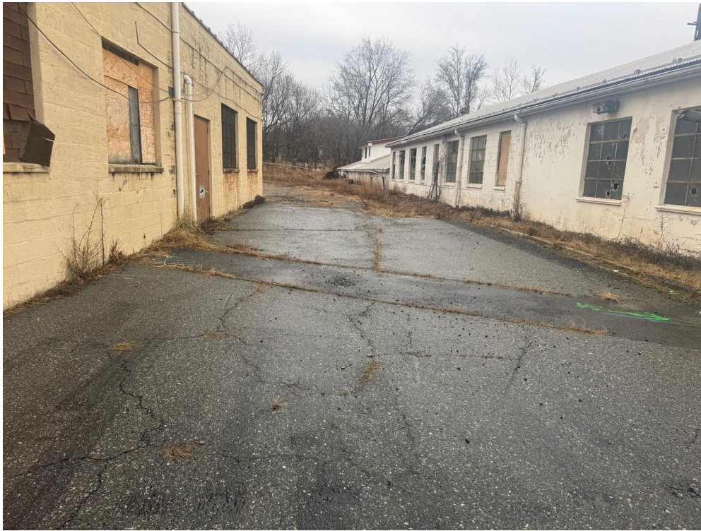
A view of the area between Building A (tan) and Building B (white). The façades of the buildings are damaged, and windows are either broken or boarded up.
