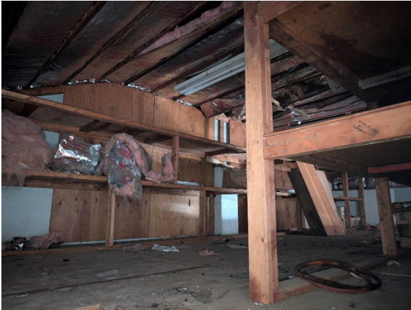
A close-up view of top level of the loft where trash and debris can be found.
