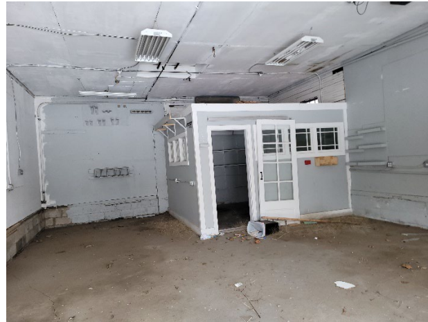
Above Right: Another view of Building D's interior that shows trash and debris on the ground.
