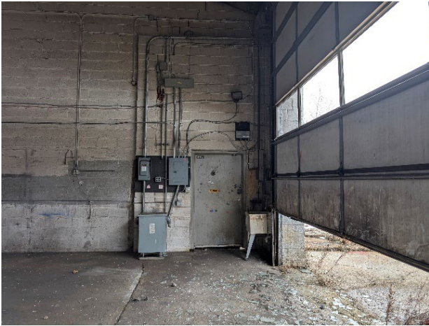
View of one of the garages with a broken door.
