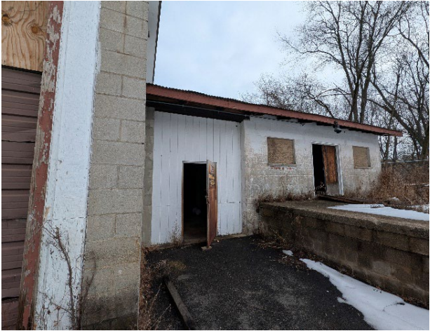
Additional rear entrances to the building with boarded-up windows.
