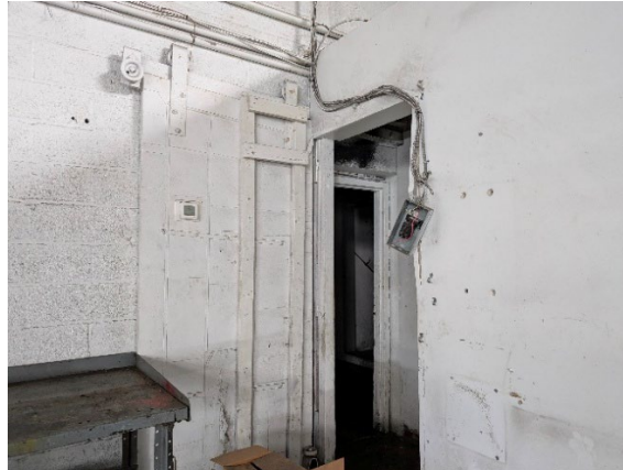
View of the doorway in Building A leading to the bathrooms. Also pictured is the exposed wiring.
