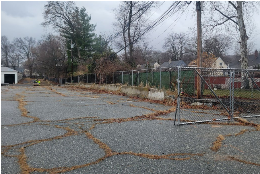
Another view of the gate at the entrance to the property. The pavement is cracked and overgrown, and parking is undefined. As seen in the above image, the site slopes downwards towards Building E.
