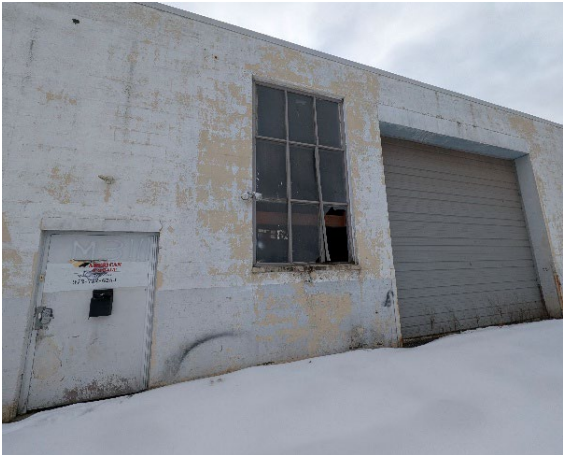
View of garage door and broken window.
