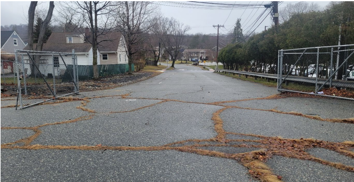
View of the asphalt driveway which provides access to the site from Grove Avenue. The site visit on March 12, 2026, clearly reveals the dilapidated condition of the pavement.
