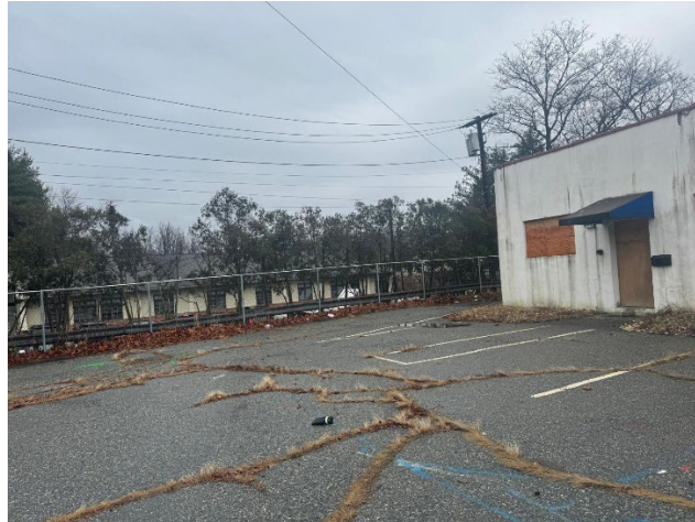
Additional view of Building A and fence along the northerly property line depicting the dilapidated building and parking area.
