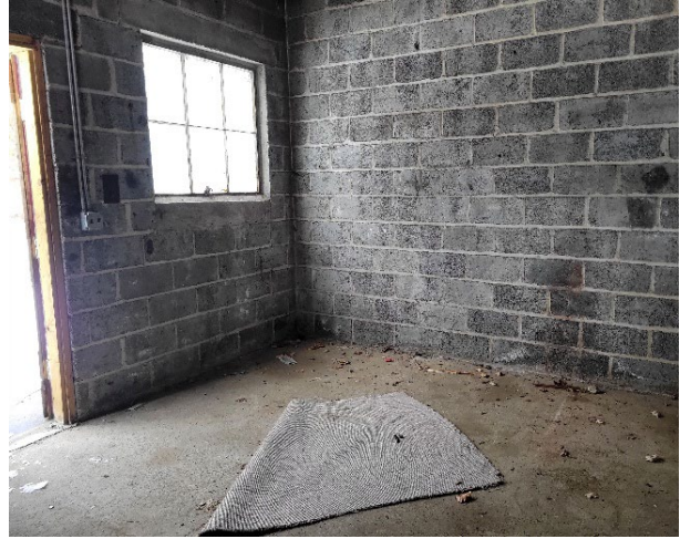
Additional image of the interior showing further signs of mold and water damage to the physical structure.
