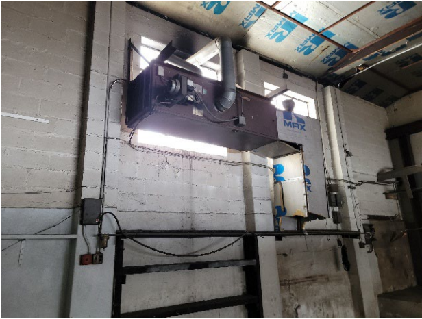
View of an AC unit in the third garage bay.
