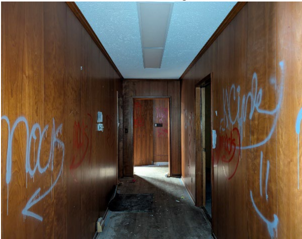
Evidence of vandalism and graffiti that could be found all over the hallways to the offices.
