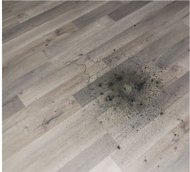
Close-up view of ashes and soot.
