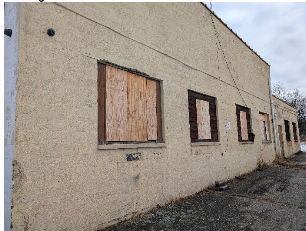
View of more boarded-up windows on the side of the building.
