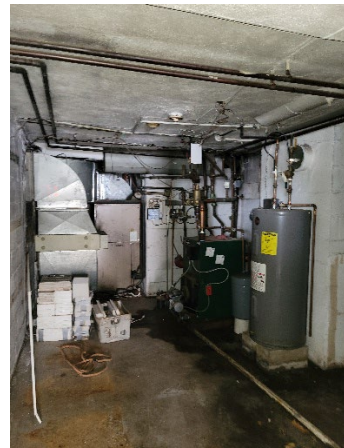
Utility equipment that could be found in Building B.
