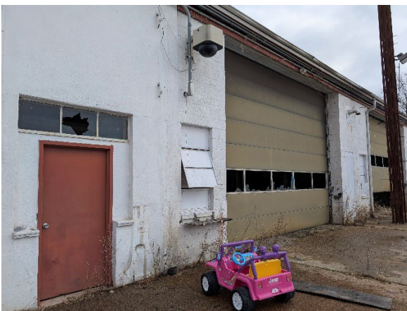
View of the rear entrances to the building with broken windows and an abandoned toy car.
